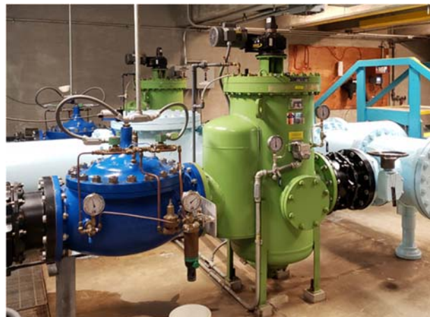
Exhibit 2 - Blue Lake WTP Strainers and Pressure Reducing Valves
