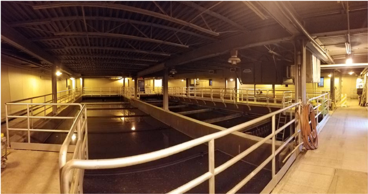
Exhibit 11 – WWTP Primary Clarifiers
