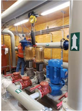
Exhibit 10 - Whitcomb Heights Pump Station
