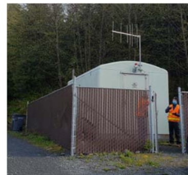
Exhibit 9 - Hillside Pump Station
