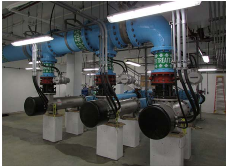
Exhibit 3 – UV Disinfection Facility
